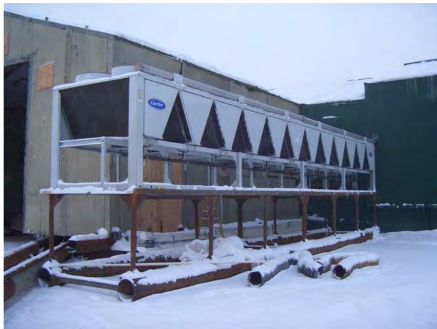
Figure 13. Air Cooled Condenser for ORC#2
