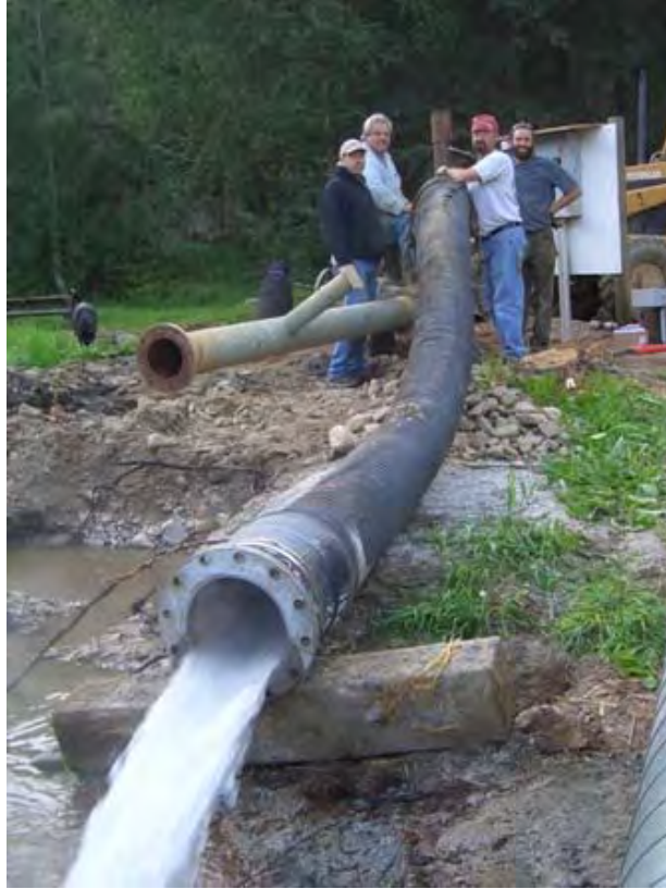
Figure 16. Geothermal well pump tested prior to hookup to pipeline
